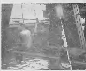
An important day for Aruba and Lago. The last pile of the new No. 3 Finger Pier is driven, marking a vital point in the construction of the pier. Two Netherlands Harbor Works men manipulate the ropes which control the hammer of the pile driver, "Araba".
